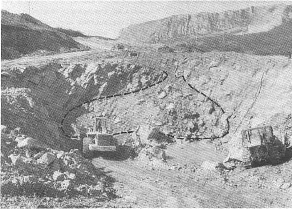
Fig. 5.- Wedge failure ( w_1 ) on the West face of the excavation
