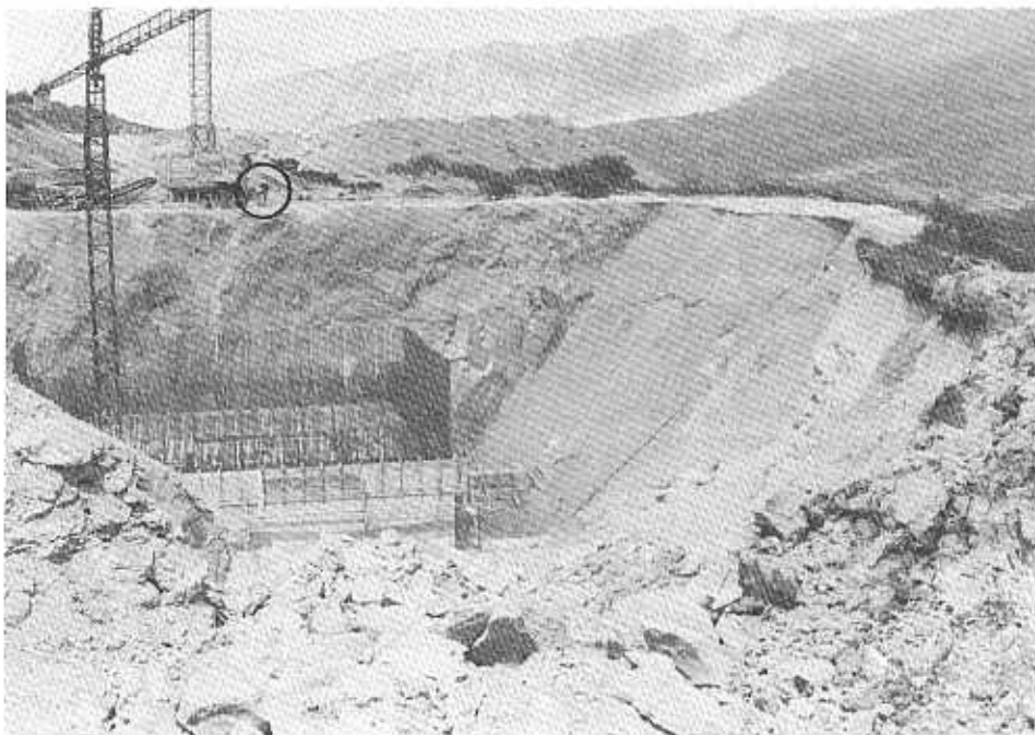
Fig. 6.- Plane failure (P2) on the North face of the excavation (see man in the circle for scale).
